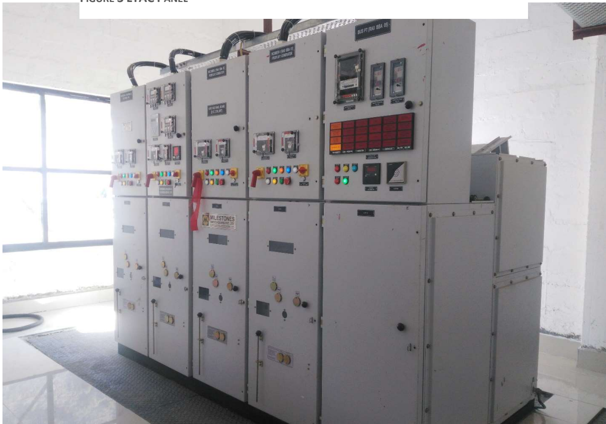
FIGURE 4 MV SWITCH GEAR PANEL
