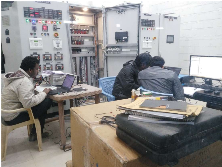
FIGURE 2 SCADA SETUP AND GENERATOR PROTECTION TEST INSIDE CONTROL ROOM
