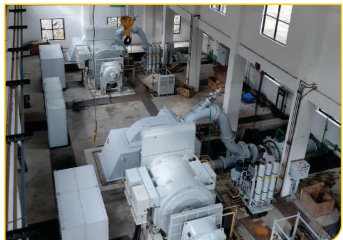
RUDI A Turbines and Generators
