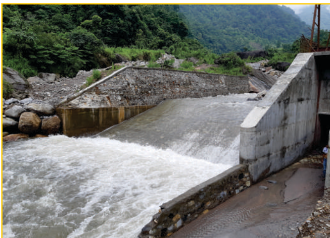
Rudi A Headworks during moonsoon
