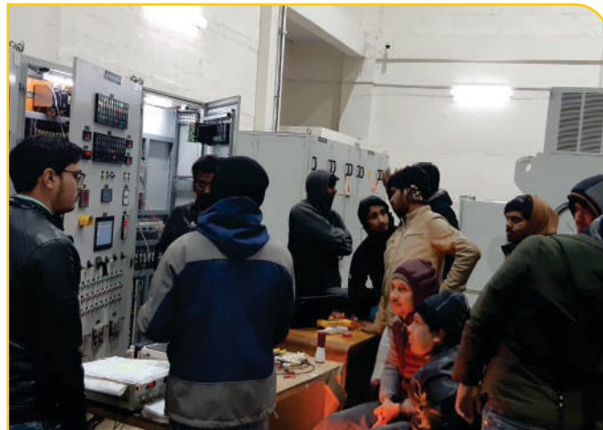
Pre-commissioning tests at Rudi B Powerhouse with NEA Officials
