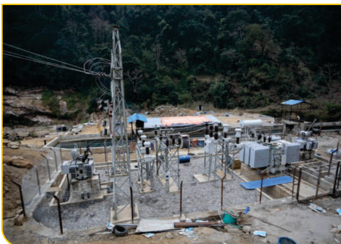
Rudi A switchyard
